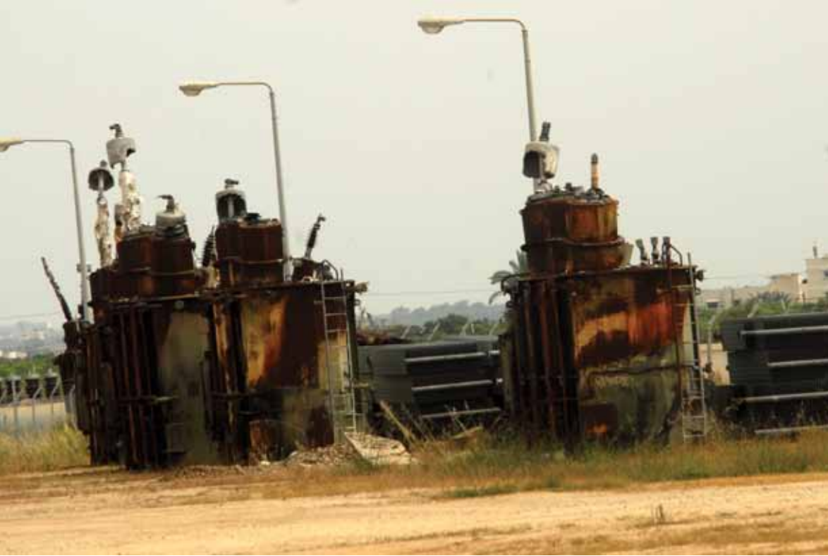
The Gaza power plant was damaged after being bombarded by Israeli forces. (2009)
